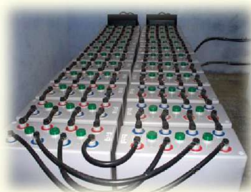
Local Operator of Biogas Engine
