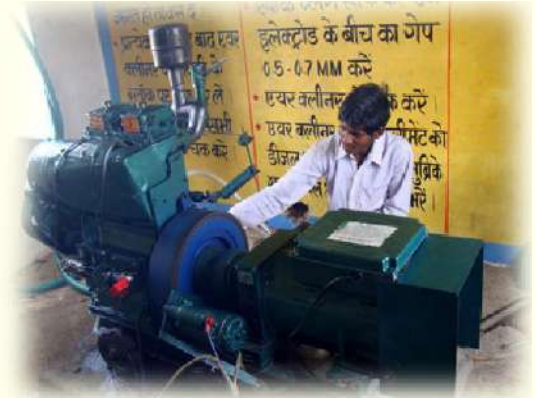
Local Operator of Biogas Engine
